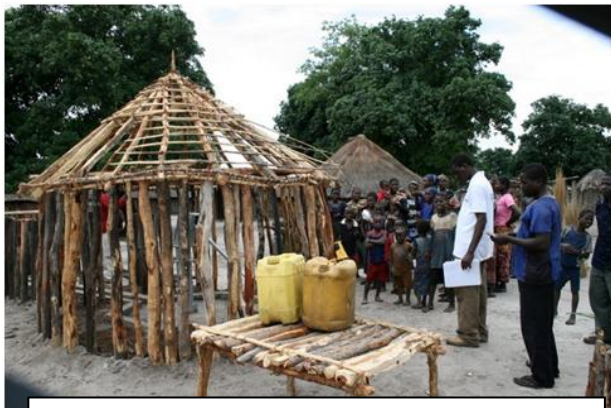
Completed pump with pump house walls and unfinished roof and jerry can stand
