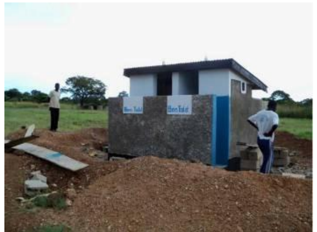
Set of Latrines in a Kaoma School
