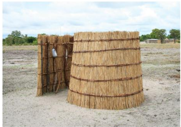
Another type of latrine constructed from local materials – a roof will go on before the rainy season
